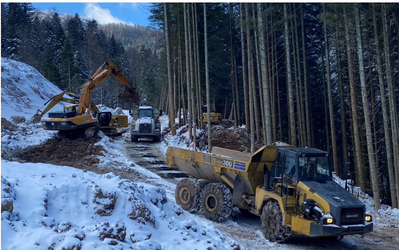
Figure 2: Site clearing and construction of the access road to the lower and upper portals
