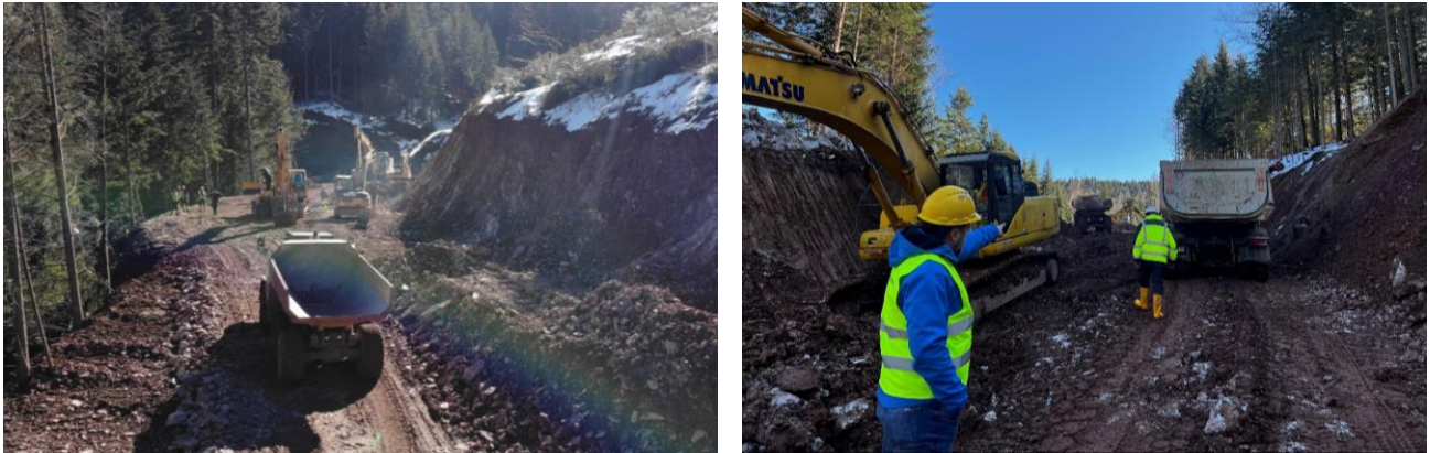
Figure 1: Site clearing and construction of the access road to the lower and upper portals
