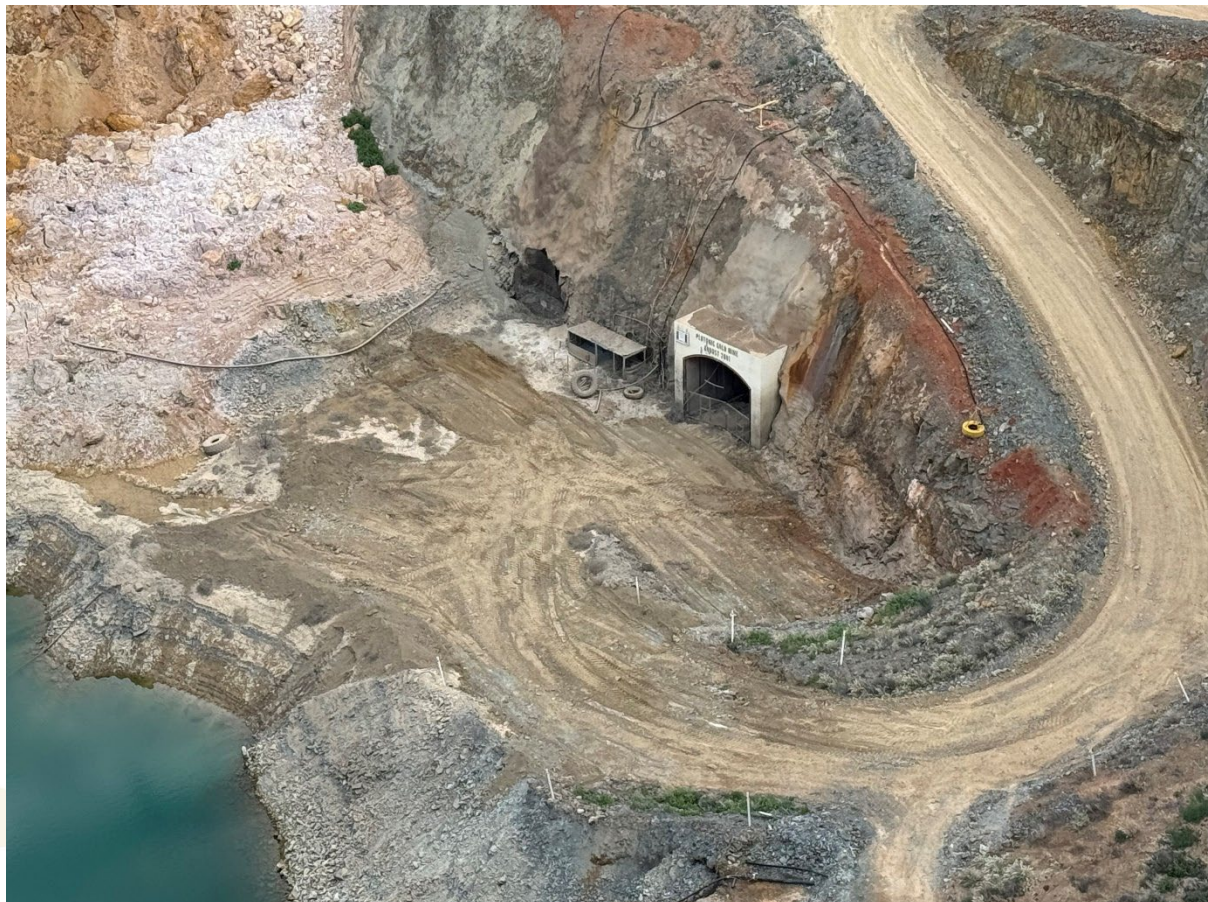
Figure 3: Plutonic East portal location at base of open pit showing refurbished access
