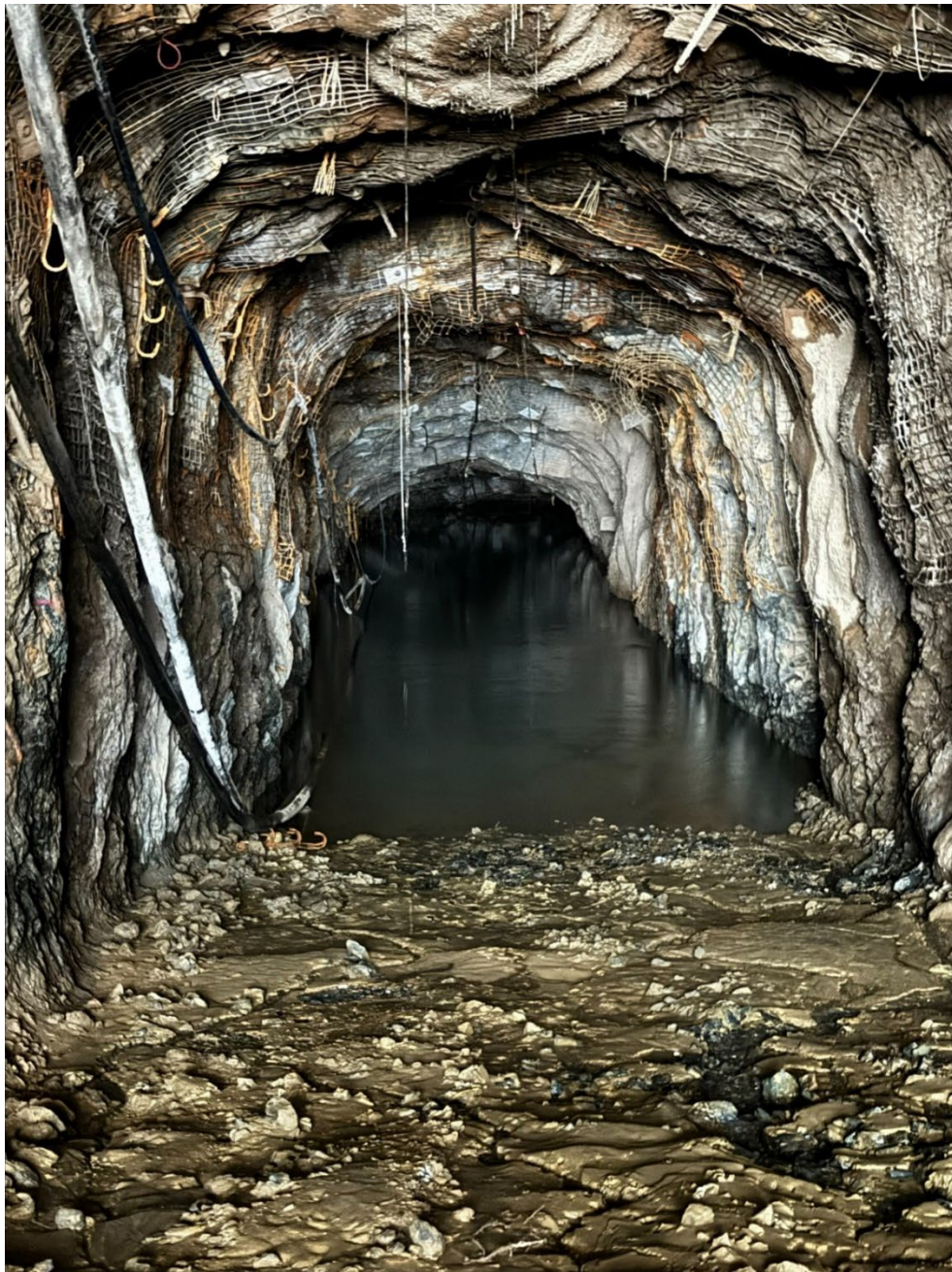
Figure 6: Plutonic East decline dewatering
