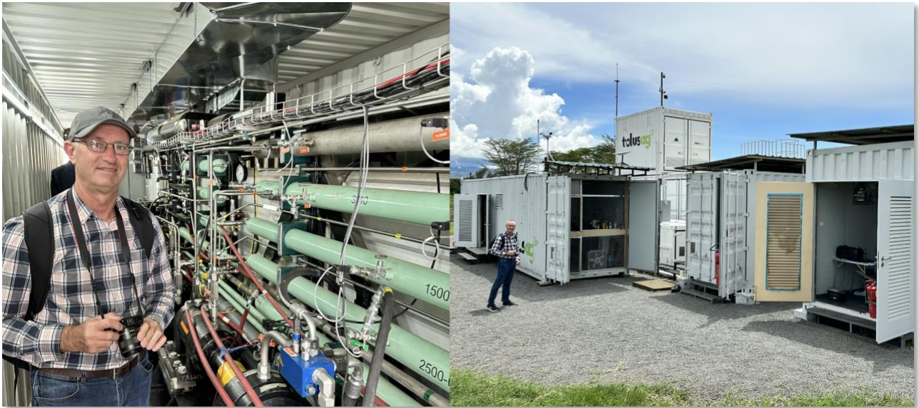
Figure 3 – Minbos COO Steven Abbott on site at the Talus Kenya site, inspecting their modular green ammonia project.
