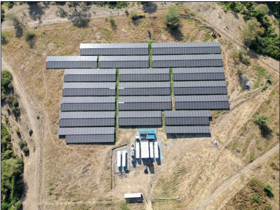
Figure 2 - TalusAg Green Ammonia Project, powered by Solar Energy, located in Kenya.
