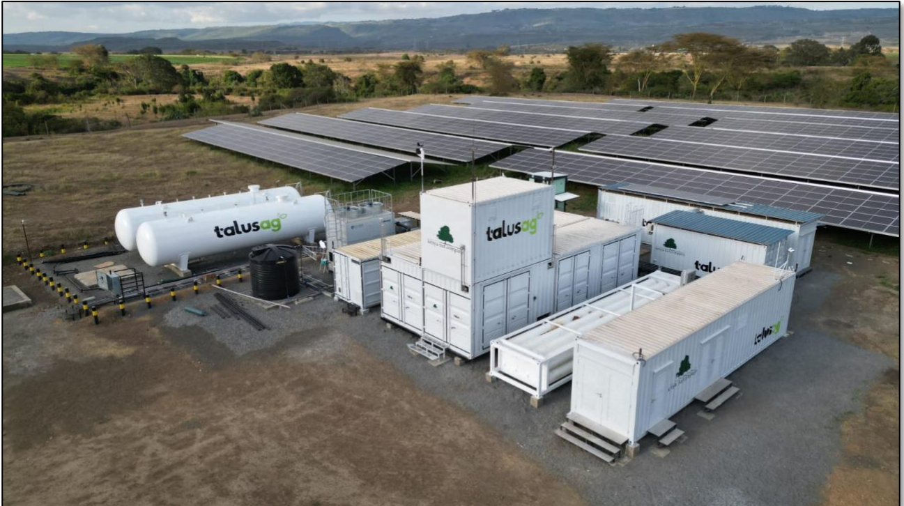
Figure 1 - TalusAg Green Ammonia Project, powered by Solar Energy, located in Kenya.
