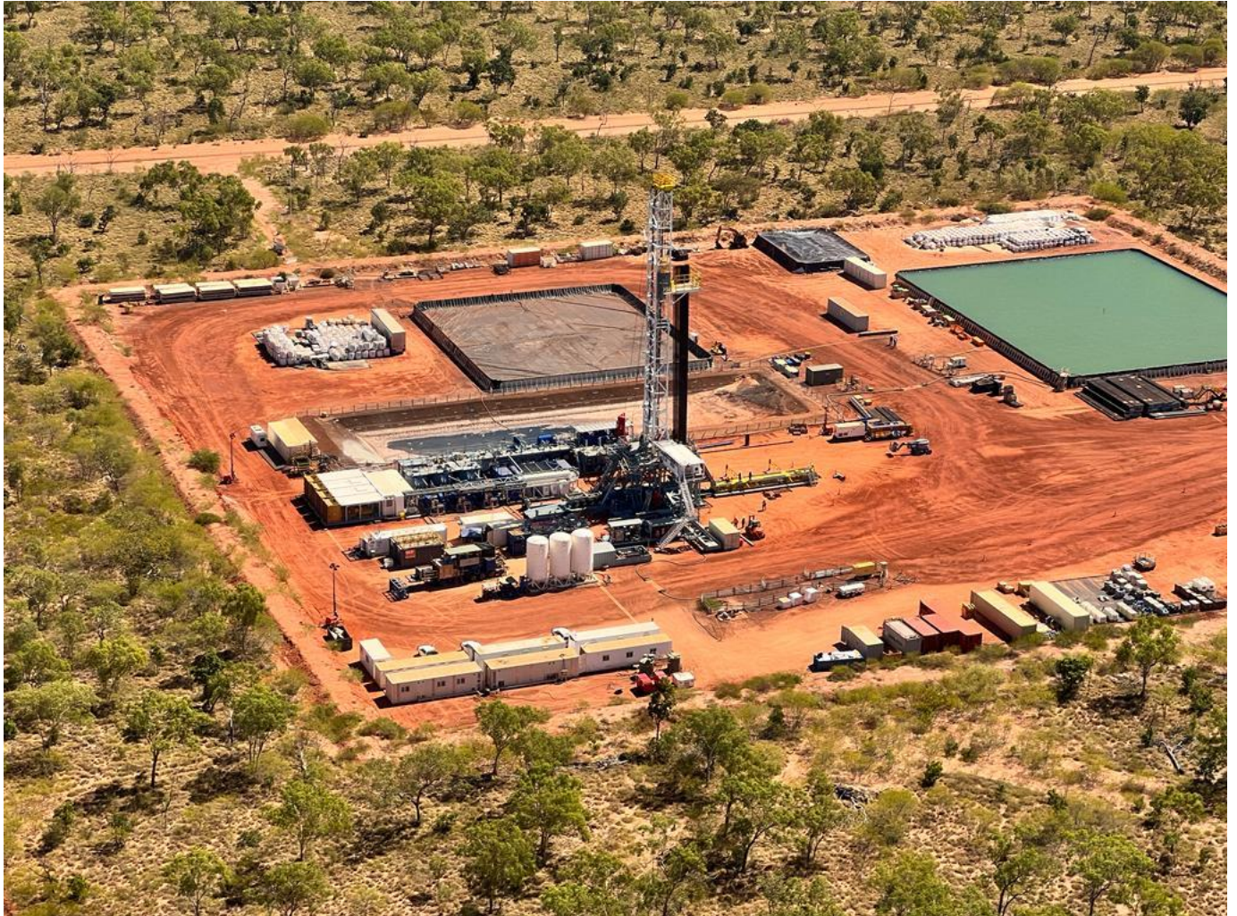
Figure 1: H&P's super-spec FlexRig® Flex 3 Rig mobilised to the Shenandoah South well location.
