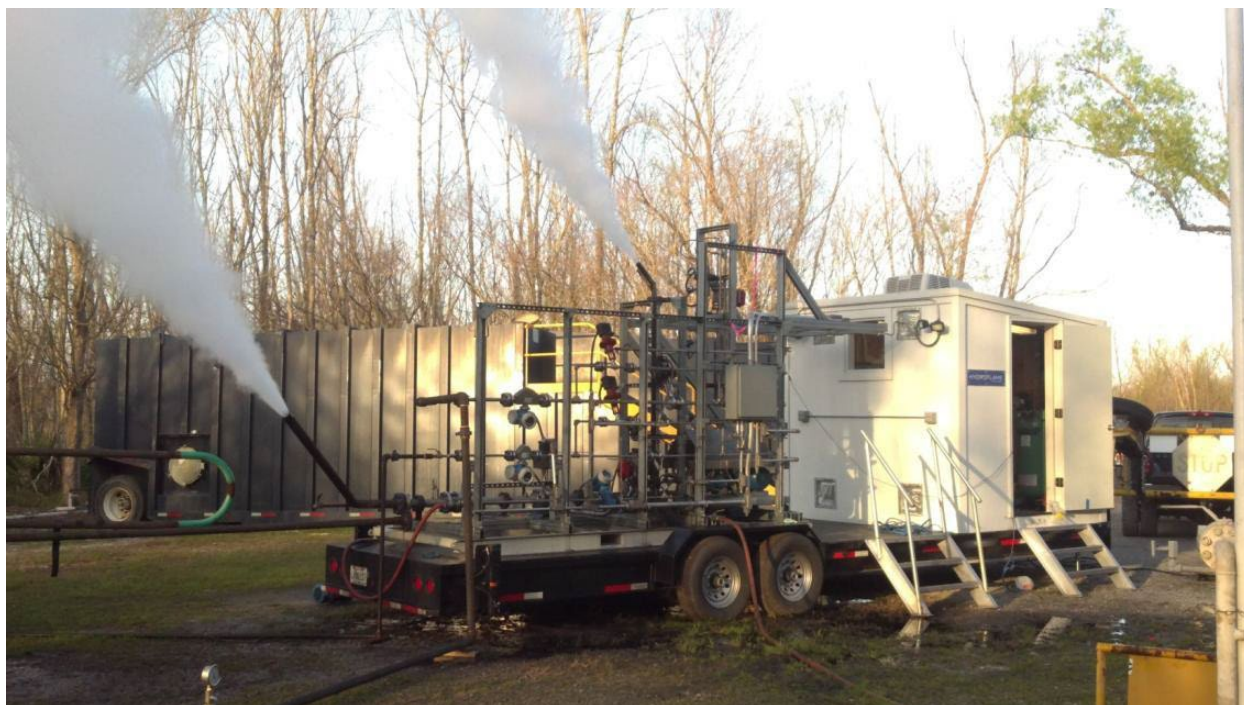
AVS' Superheated Steam Generator
