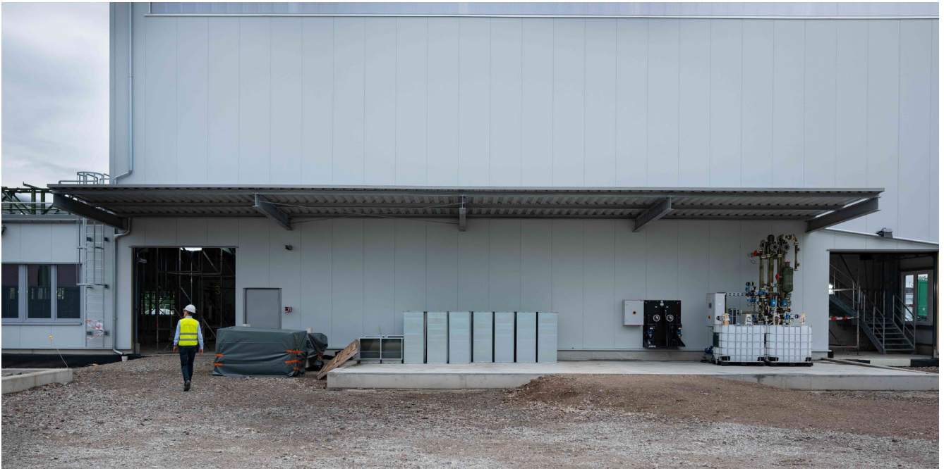
Figure 3: Vulcan's constructed Lithium Hydroxide Optimisation Plant
