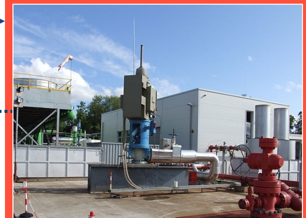
Geothermal Plant - Landau
